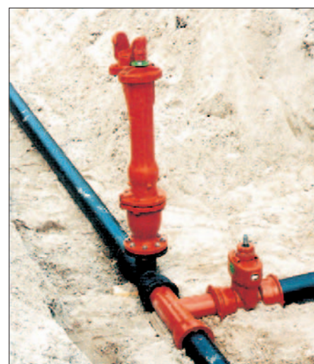
Fig. 8: Hydrant assembled directly above cast-iron mains
