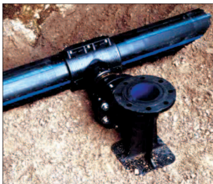
Fig. 10: Combination of PE fitting and cast-iron ducks-foot bend
