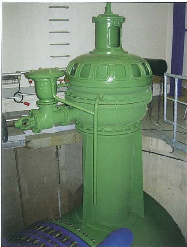
(c) Existing DN 900 air valve for venting the DN 2300 outdoor pipeline to the Schwammenauel hydropower station.
