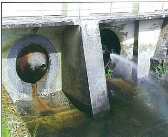
(b) Far right: A RIKO DN 250 plunger valve with venting set in the bypass, above the EKN DN 2300 butterfly valve with a brake and lift cylinder.
