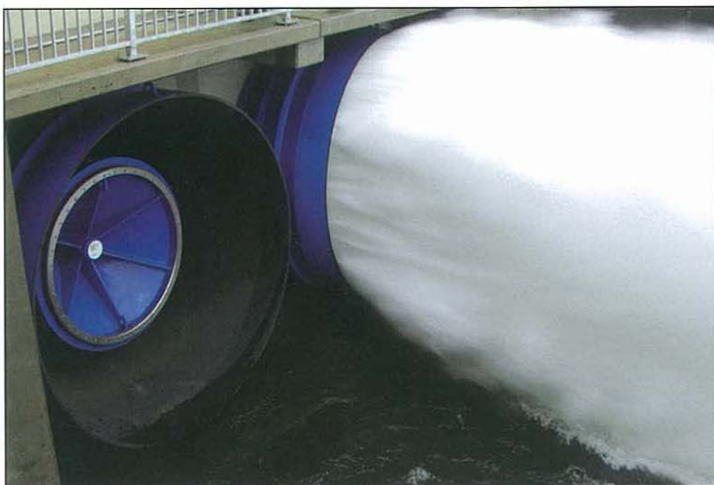
The DN 1800 hollow jet valve for the left bottom outlet during the first set-up.
