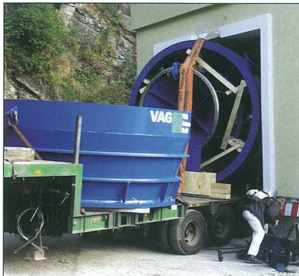
(d) Delivery of the first DN 1800 hollow jet valve, pre-assembled in the wall pipe, together with the associated guide pipe during entry into the gate valve house.
